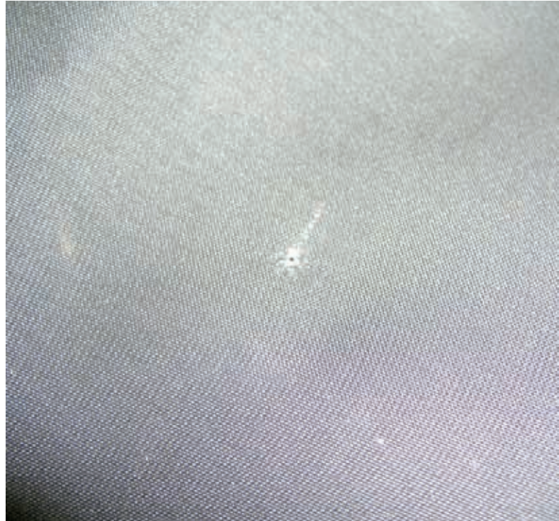
A tear in the support frame caused by external mechanical influence
